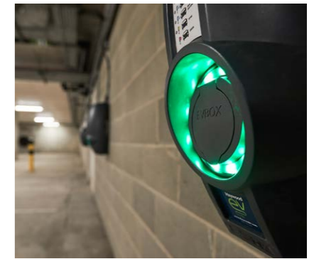
Electric car charging points
